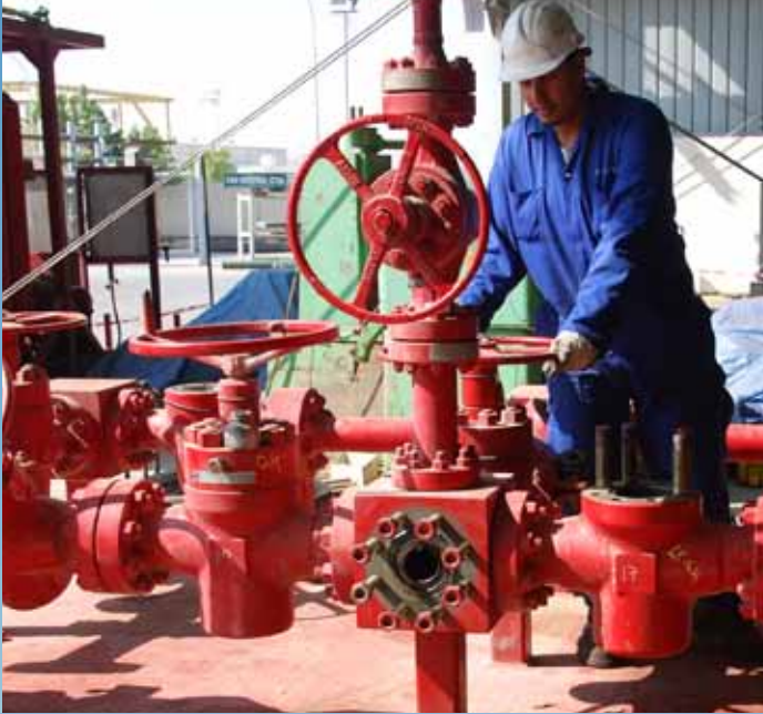
CHOKER MANIFOLD MAINTENANCE
