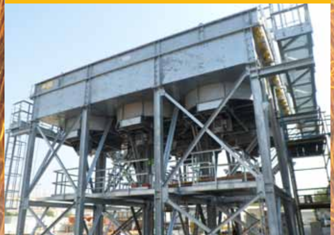
AIR COOLED HEAT EXCHANGERS
